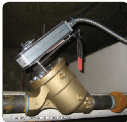
Owners of the 271 building replaced each air-handling unit chilled-water control valve with a precision control valve.
